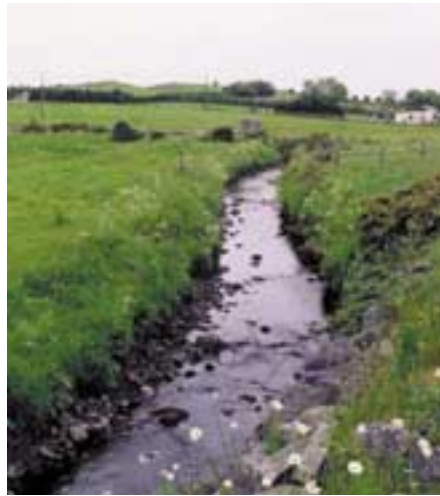
Arterial Drainage Damage
